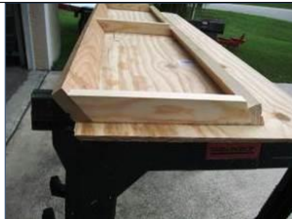
The lower angle of 130° is achieved with a 40° cut along the forward facing edge of the lower cross piece. Note that the bow bottom has also been planed to an angle. The upper cross piece is cut at 27°. The uprights are cut at similar angles.
